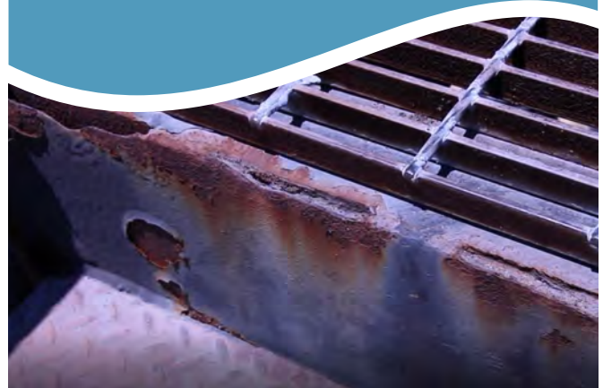
Existing Wastewater Treatment Plant – Bastrop, Texas
